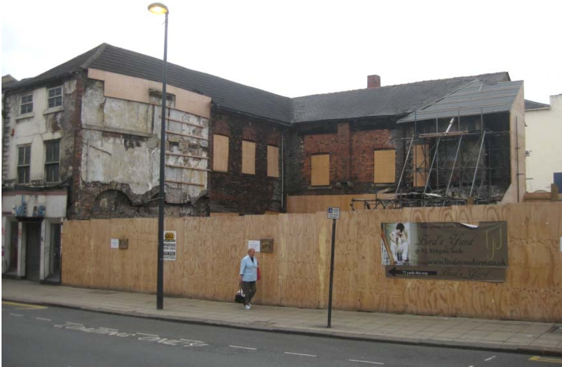
The First White Cloth Hall today following demolition of the west wing. Temporary repairs have been carried out to ensure that the structure is watertight , secure and stable.
